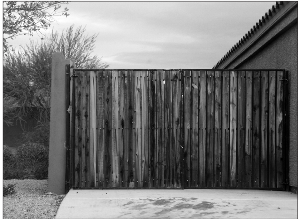
Restaining and sealing wooden gates can add years of life to the wooden slats. The harsh desert sun and temperatures can cause untreated wood to dry rot.
